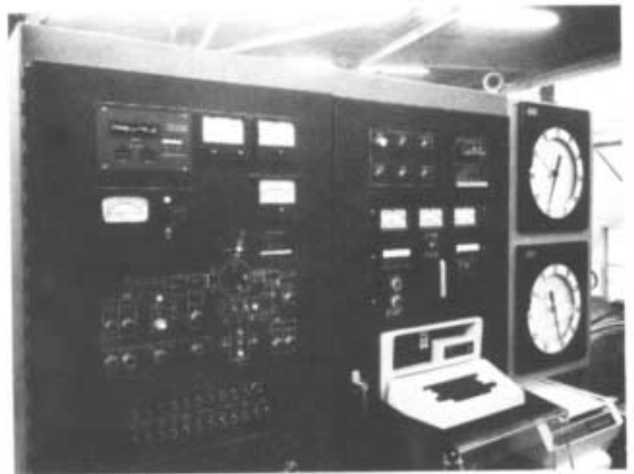
Figure 16 - Vacuum Precision Casting Furnace operator's control station with microcomputer.
