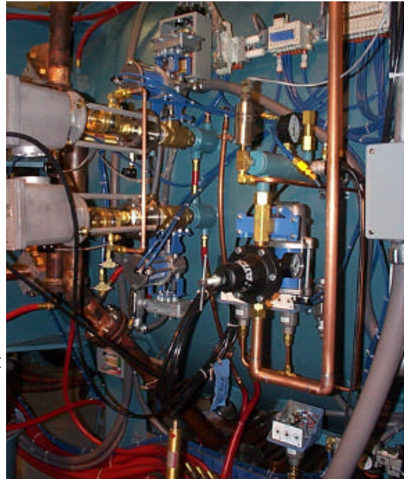
Photograph of C/VI furnace chamber showing gas regulators on backfill line with 3 position U/E pressure switches, and chamber overpressure pressure switches.
