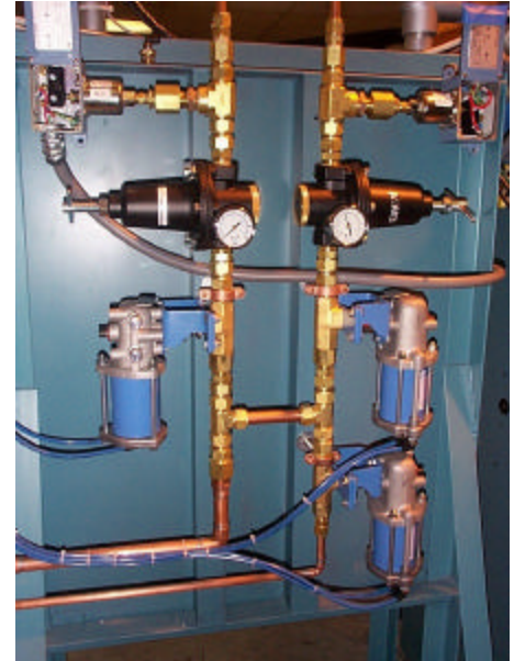
Photograph of C/VI gas panel with pressure
