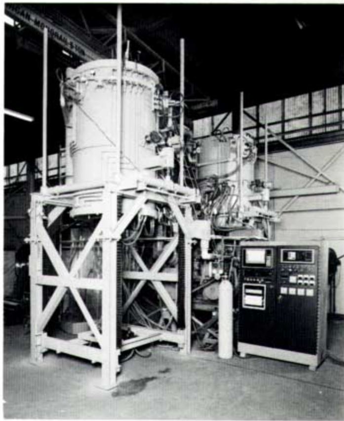
Fig. 2. Typical Vertical Elevator Hearth CVD Furnace
