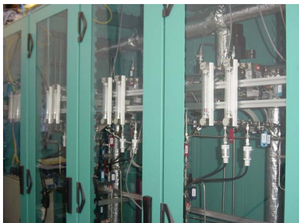
CVD Inert and Process gas cabinet with Mass Flow Controllers.
